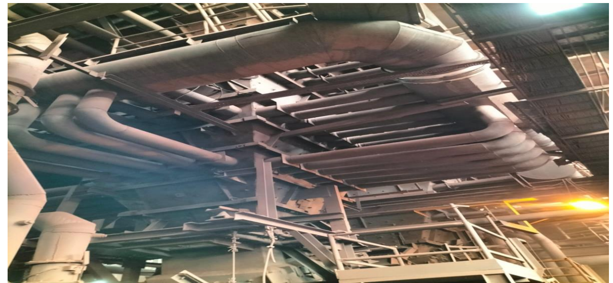
Nozzle arrangement at the Bunker
