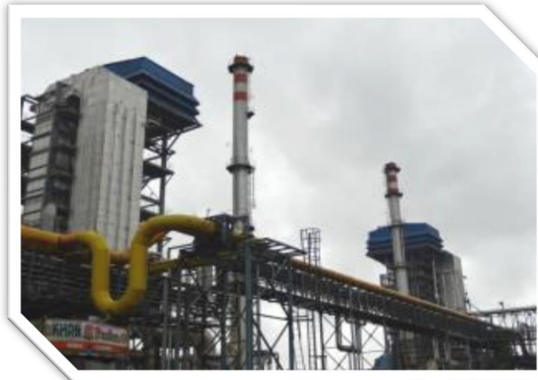
WASTE HEAT RECOVERY POWER PLANT
